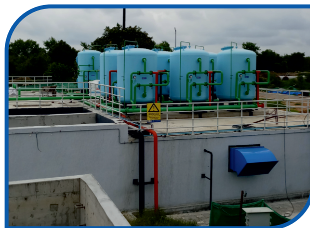
SEWAGE TREATMENT PLANT
